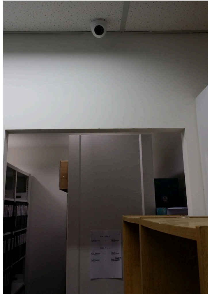
Unsecured room with personnel files
